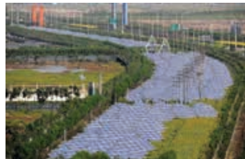
PV Power Generation Project in Central Avenue
