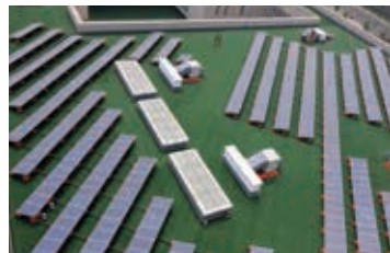
Distributed PV Project in Amine Industrial Park
