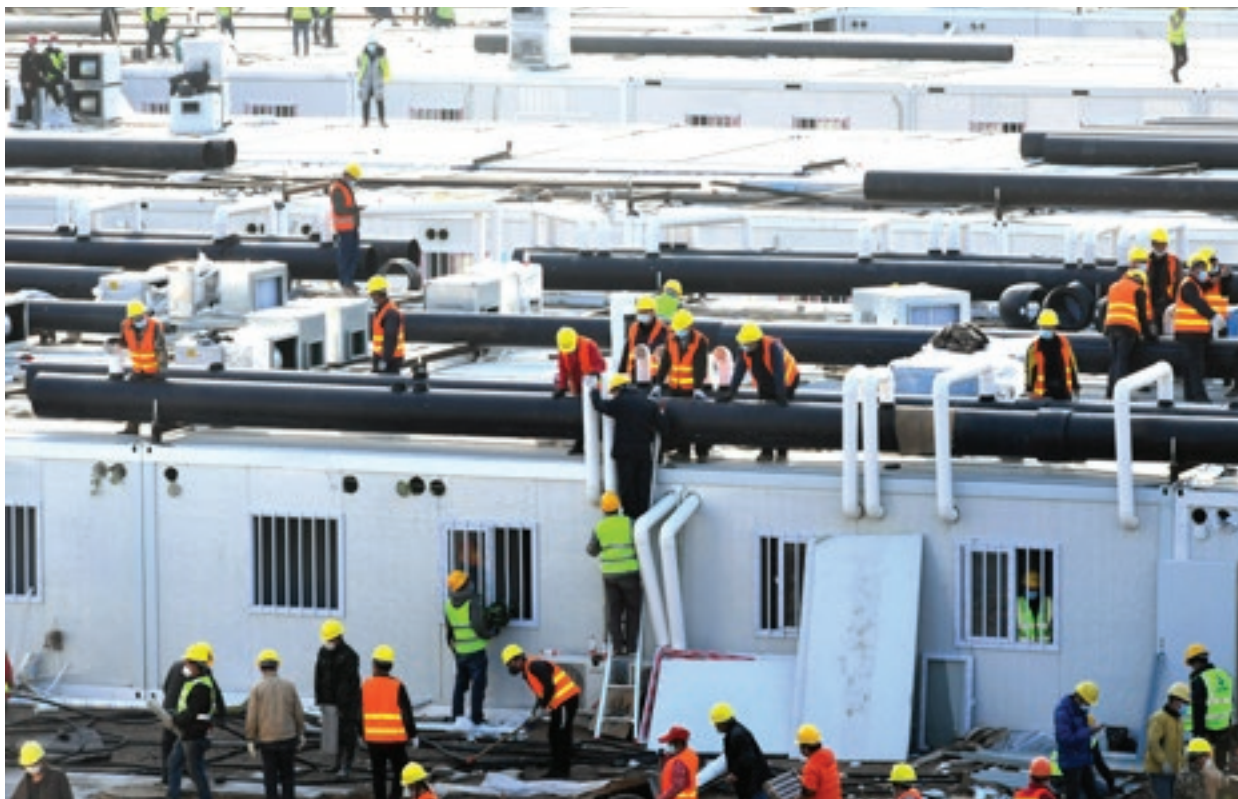
Workers at the construction site of Leishenshan hospital in February 2020. Image: An Yuan / China News Service via Getty Images
