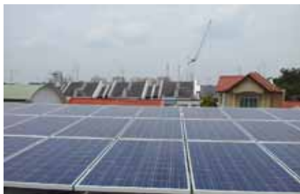
Rooftop installation at Poh Huat Crescent, Singapore
