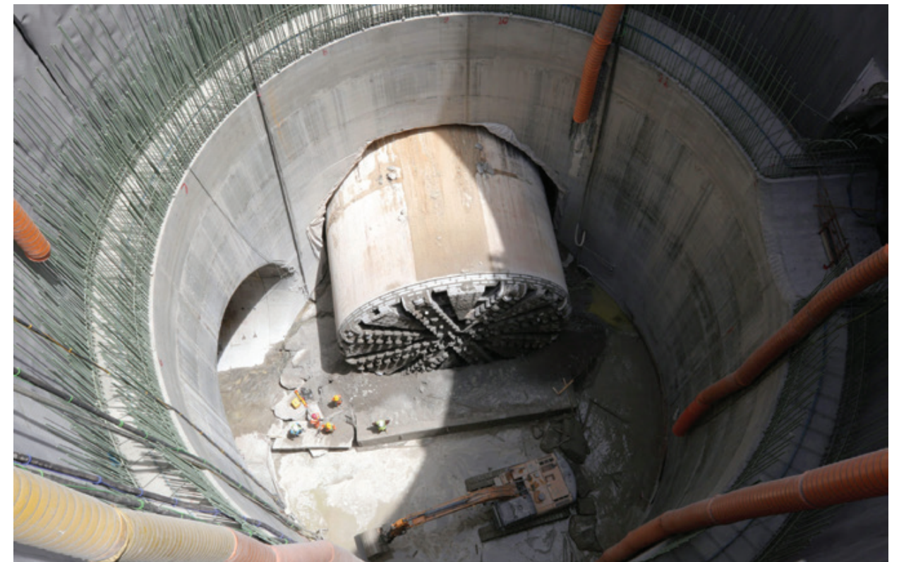
The tunnel is a groundwater and stormwater collection network, running 45 m deep. Image: Government of Dubai
