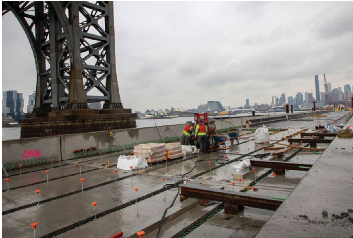
Construction of elevated East River Park as part of the ESCR project along the East River in lower Manhattan. Image: NYC Department of Environmental Protection
