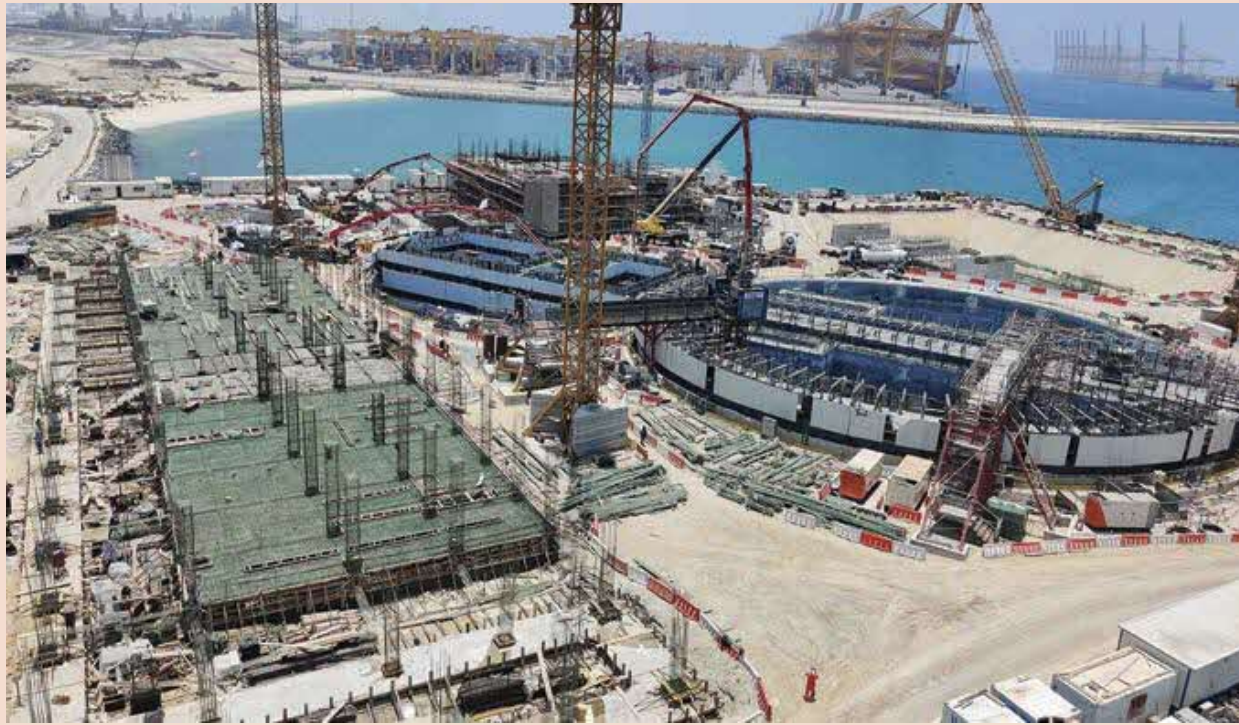
The Dubai Deep Tunnel Storm Water System can drain 40% of the entire urban area of the city. Image: Stantec
