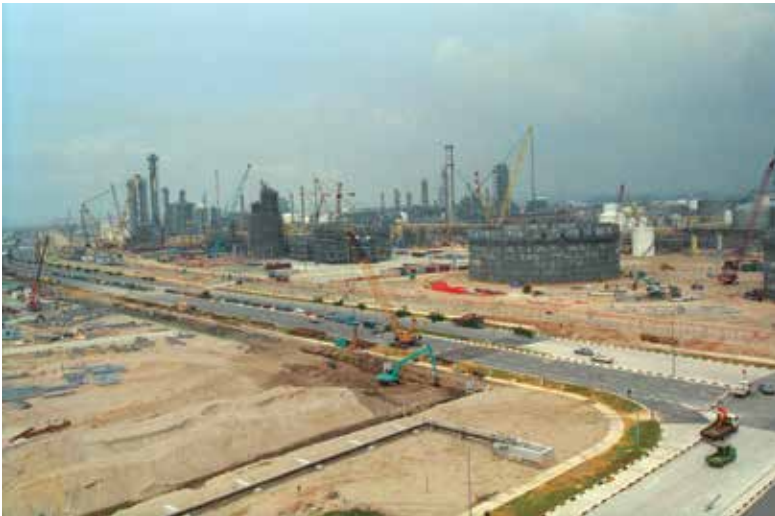
9. View of land reclamation works in progress at Jurong Island, taken during the launch ceremony of Jurong Island's amenity centre Oasis@Sakra and internet portal JurongIsland.com.
