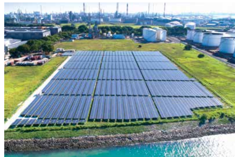
24. Aerial view of the SolarLand installation on Jurong Island. The system is modular and flexible, allowing JTC to maximise land that is temporarily vacant and to deploy the land when needed.
